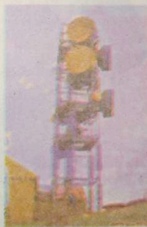
Figure 15.30: Microwave relay station
